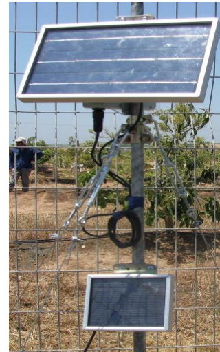
Transmitting modem behind solar panel
